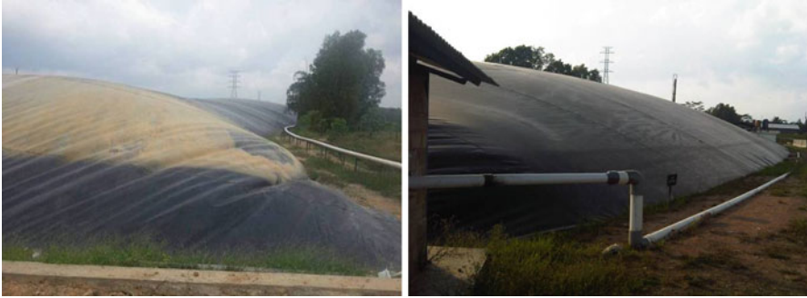
Fig. 22.2 An installed balloon-type anaerobic digester
