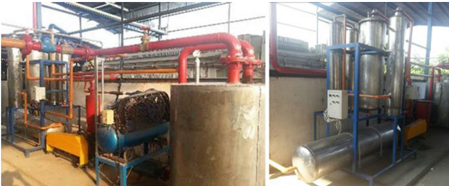
Fig. 22.3 Installed biogas purifier system
