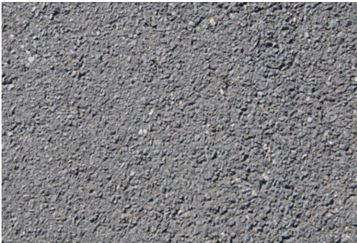
Fig. 8.3 Aggregate of service lane of Dorset Road, Bayswater, at location of testing
