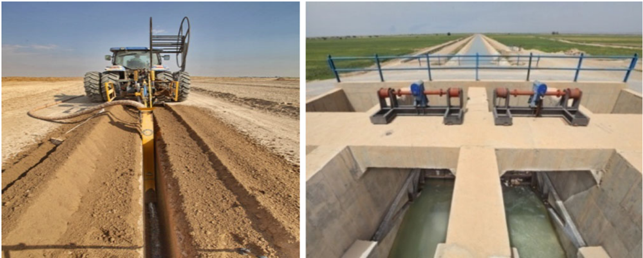
Fig. 7.44 Drainage and irrigation systems are being installed in saline soils (Typic Torrfluvents) of Dashte Azadegan, west of Khuzestan plain (Courtesy by Dr. N. Ebrahimi)
