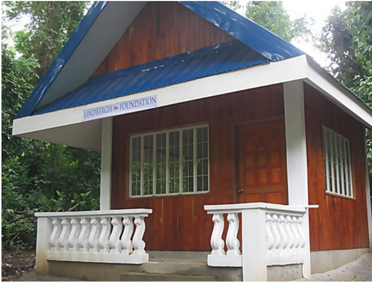
Fig. 10.3 A small wooden house protected underneath by lahar barrier remained free of subterranean termites 7 years after construction
