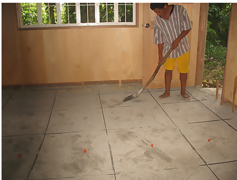
Fig. 10.2 Installation of lahar barrier underneath floor and foundation walls prior to the pouring of concrete
