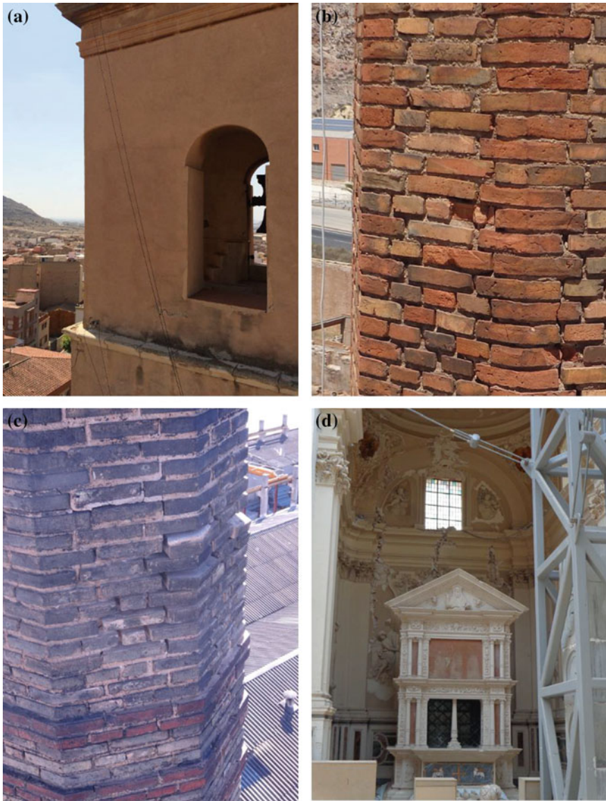
Fig. 1 The most frequently observed pathologies in built heritage: a discoloration, b spalling, c mortar loss, d cracking
