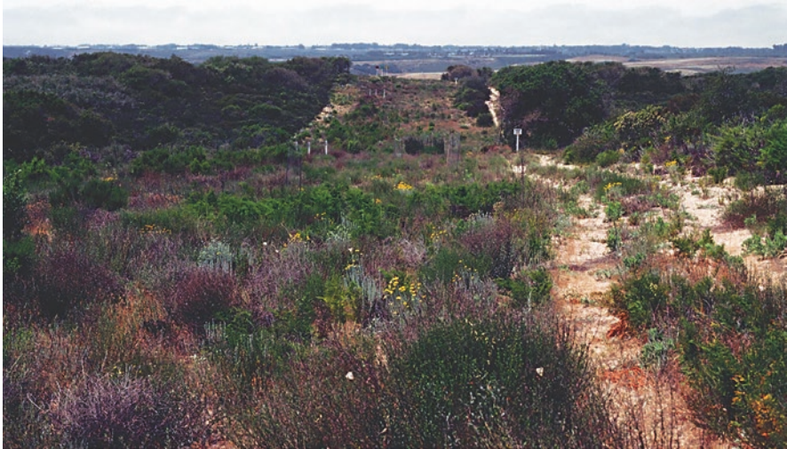
Fig. 13.4 Vegetative cover in second growing season of pipeline revegetation project. Topsoil was conserved during construction and replaced and many unseeded natives recovered from the seedbank. Most species visible here are short-lived perennials or sage scrub species. Surrounding vegetation is 50–60-year old chaparral on sandy soils (D’Antonio and Howald 1990). Burton Mesa region, Santa Barbara County. Photo by Carla D’Antonio
