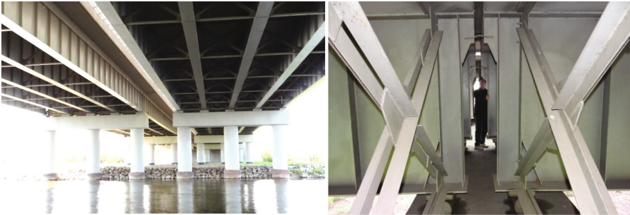
Fig. 2. Investigated bridge: (a) bottom view of superstructure, (b) view of intermediate support area
