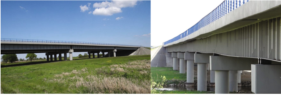
Fig. 1. Side view of investigated bridge – visible excessive permanent deflection of superstructure
