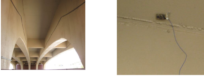
Fig. 5. Accelerometer sensors installed on the bridge.
