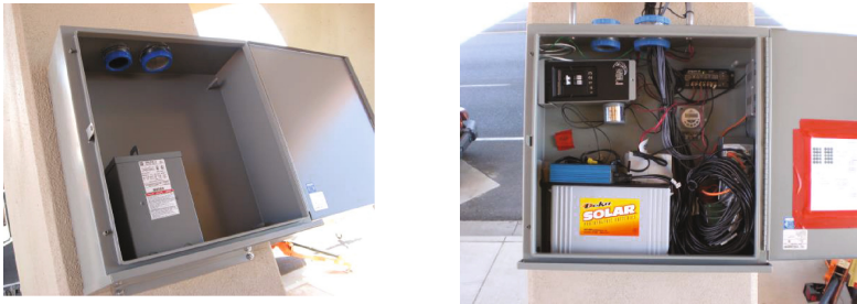
Fig. 4. Steel box used for the data acquisition device housing.
