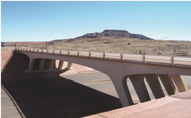
Fig. 2. K-frames of Bridge 7937.
