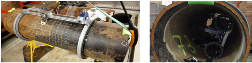
(a) Exhumed pipe on which internal and external measurements were performed. (b) Pipe assessment robot performing internal measurements.
