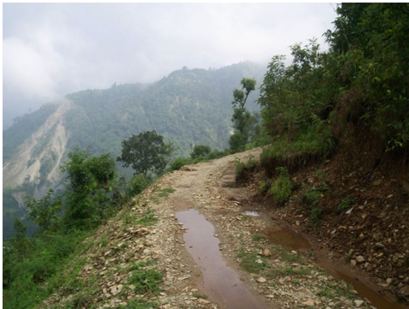
Fig. 9 Lungta's photo of the road and the landslide in the distance that now blocks access
