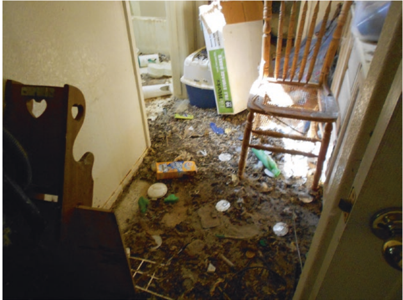
Fig. 3.16 Hoarder scene; over one inch of feces is caked to the floor in the hallway of this condominium
