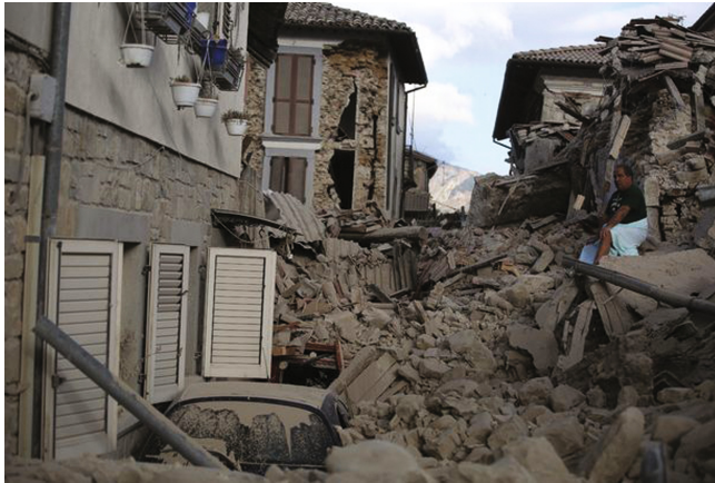
Fig. 1. Post earthquake street. Amatrice, Italy, 2016.
