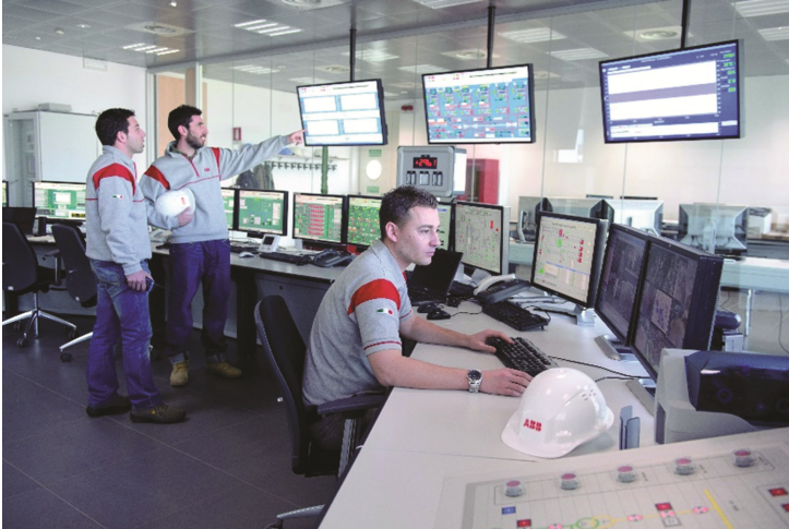
Fig. 1. Illustrative photo of a control room with operators and their workstations running applications with HMI (Source: A photo from a project)
