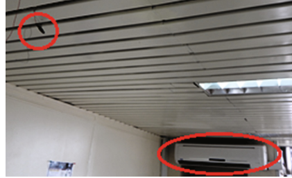
Fig. 5. Infrared transmitter and air conditioner.
