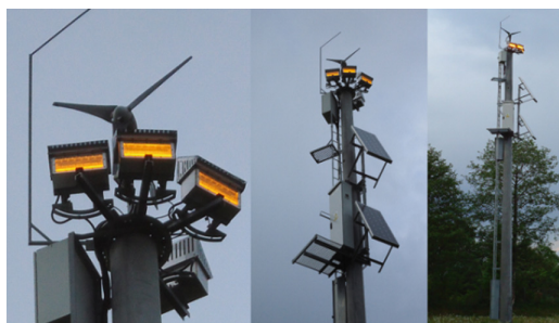
Fig. 1. The mast of warning system [own study]
