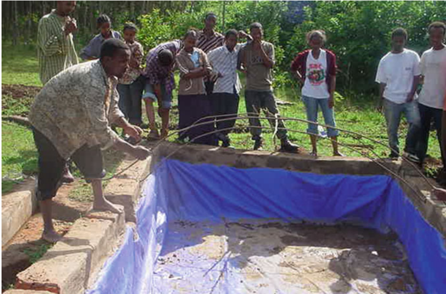
Fig. 5 Half-concrete and half-plastic lined water collection reservoir. Note the mesh wire supporting bars being installed on top of the water reservoir. Photograph Alemayehu Haddis
