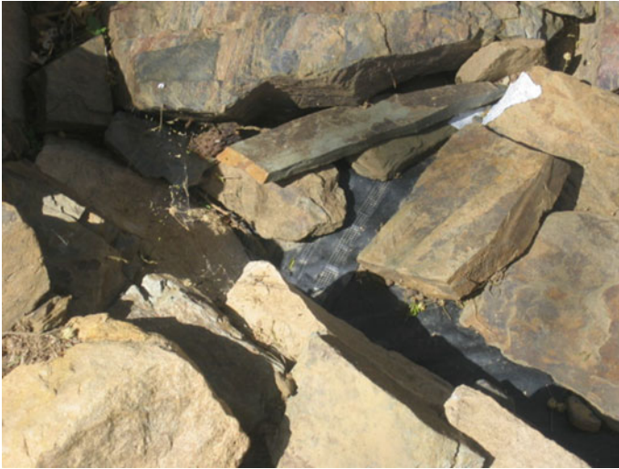
Fig. 12 Sharp edged rock riprap damages the underlying plastic liner Location: Atsbi Womberta. Photograph Gebremedhin Berhane
