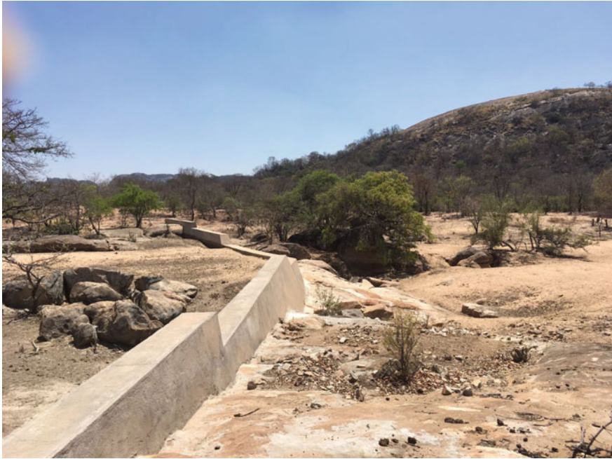
Fig. 6 A sand dam built across a river in Umzingwane, Zimbabwe. Photograph Menas Wuta
