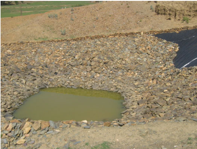
Fig. 9 Improper side slope and frequent failure of riprap. Location: Woreda: Gulomekeda. Photograph Gebremedhin Berhane
