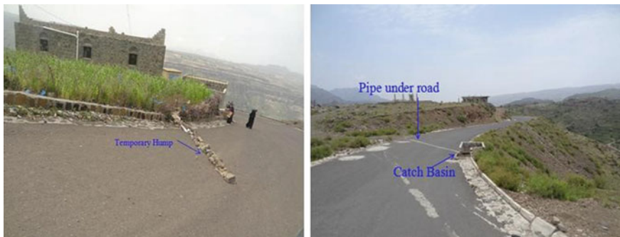
Fig. 15 Temporary hump diverting water from road surface to farmland and catch basin collecting road runoff and transporting it under the road. Photograph Mohammed Abdullah Al-Abyadh
