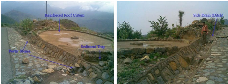
Fig. 13 Roofed roadside cisterns collecting road runoff in Yemen. Photograph Mohammed Abdullah Al-Abyadh
