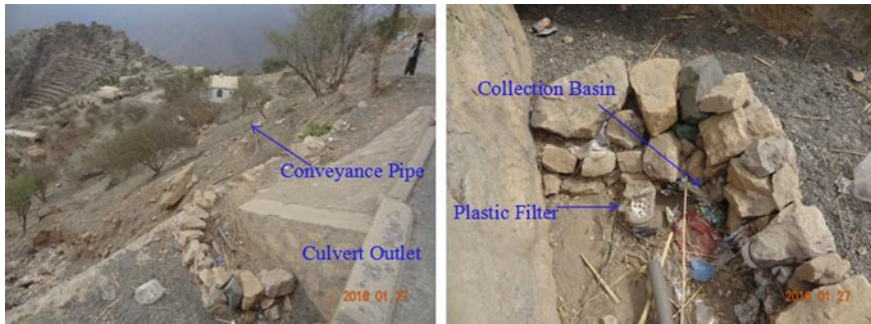
Fig. 14 Water from a culvert is gathered in a collection basin and transported through a polyethylene pipe. Photograph Mohammed Abdullah Al-Abyadh
