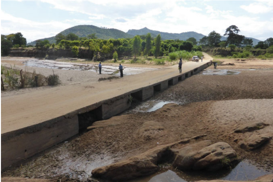
Fig. 5 Road crossing doubling up as a sand dam in Makueni, Kenya. Photograph MetaMeta
