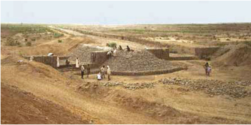
Fig. 5 Gabion flow bifurcation structure in Eritrea. Photograph MetaMeta
