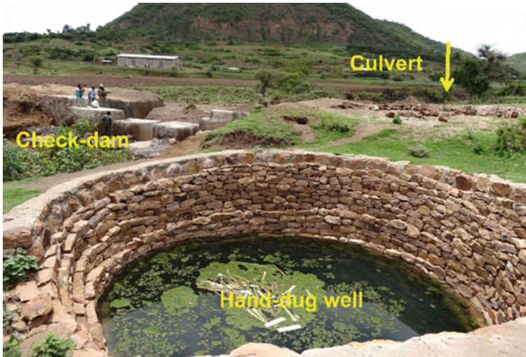
Fig. 10 Channelling water from a culvert into a check dam is enhancing groundwater in Selekleka area, Tigray, Ethiopia. Photograph Kifle Woldearegay
