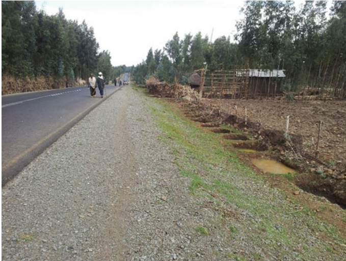
Fig. 3 Infiltration trenches along an asphalt road in Amhara Region, Ethiopia. Photograph Marta Agujetas
