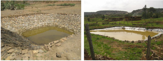
Fig. 14 Properly constructed dugout ponds [without fence (left) and with very simple wood fence (right)] from Gulomekeda and Atsbi Womberta Woredas, respectively. Photograph Gebremedhin Berhane
