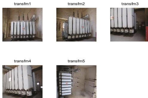
Fig. 2. The transformer pictures used as model
