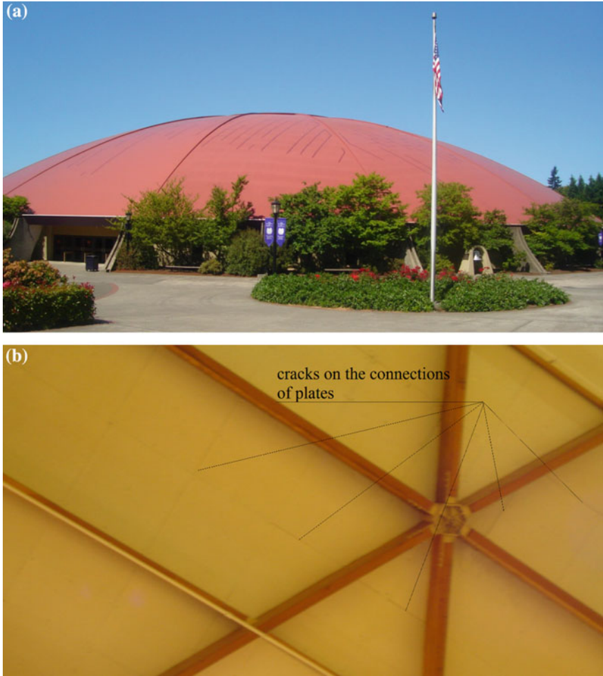
Fig. 9.21 Effects of the lowering of a node occurring in the dome in. Photographs of the authors taken in 2006, a cracks on the covering, b damage to the connections of plates around the node visible from the inside
