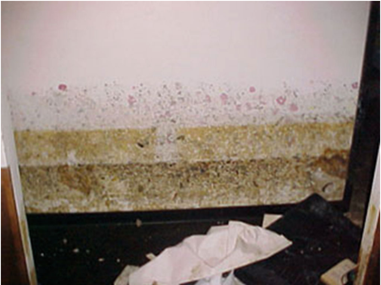
Fig. 20 Mold damage as a result of moisture wicking up drywall (Credit: Claudette Reichel – LSU Ag Center, 2005 http://www.lsuagcenter.com/topics/family_home/home/health_safety/indoor_air_quality_mold/avoiding-mold-hazards-in-your-waterdamaged-home )
