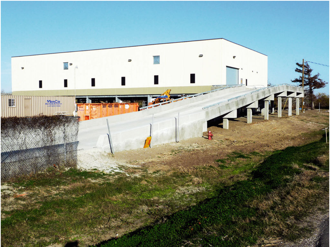
Fig. 11 Elevated warehouse under construction in Dulac, LA with ramped loading dock (Credit: LSU Coastal Sustainability Studio)
