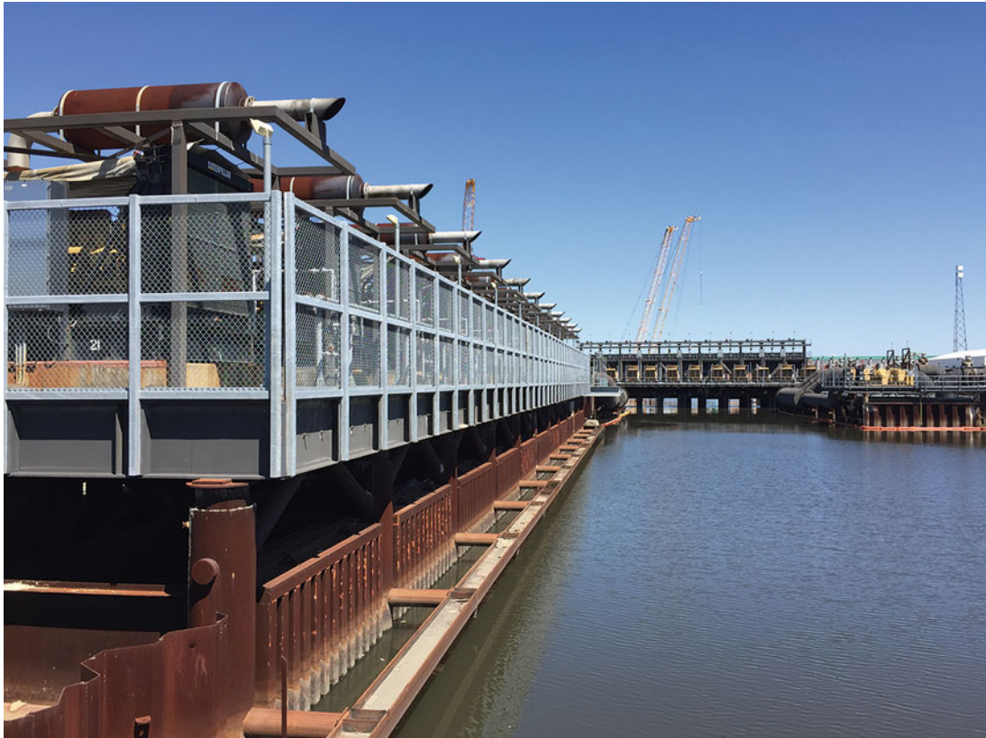
Fig. 11 17th Street Canal Pump Station (Credit: Giovanni Coakley)
