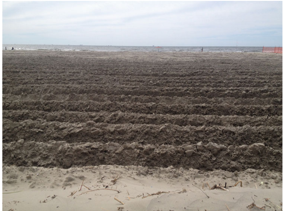
Fig. 3 Caminada Headland Beach and Dune Restoration Project (BA-45). The beach has been plowed to deter least tern ( Sternula antillarum ) nesting while the contractors await the arrival of dredged sand from a far-off shoal. Offshore oil rigs can be seen on the horizon (Photo Credit: Adrian Wiegman)
