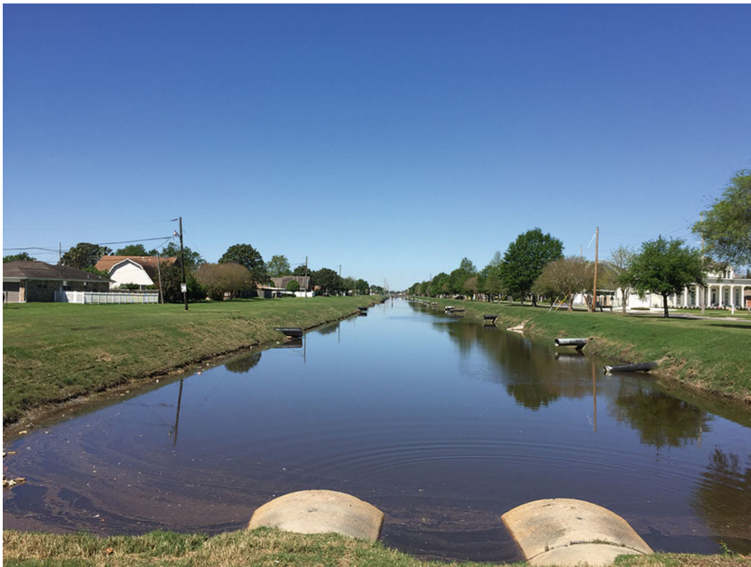
Fig. 18 The numerous drainage canals throughout the suburb of Metairie are a fact of life in these quiet residential neighborhoods (Credit: Christopher James)
