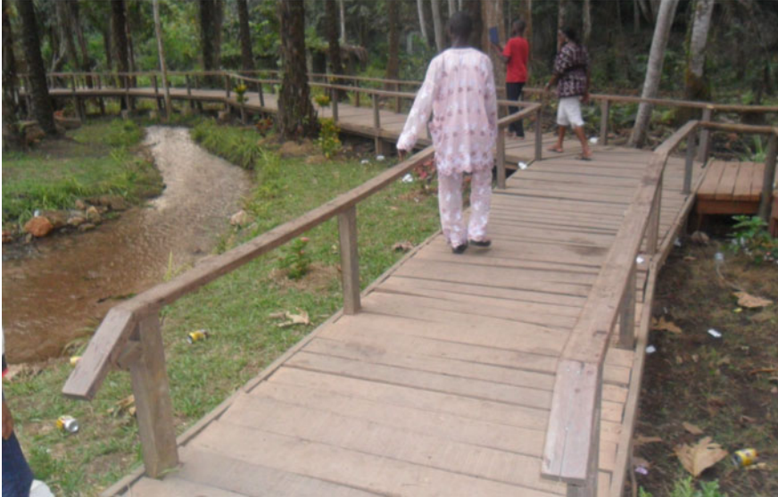
Fig. 13.2 a A shot-span wooden beam bridge. b A long-span wooden beam bridge
