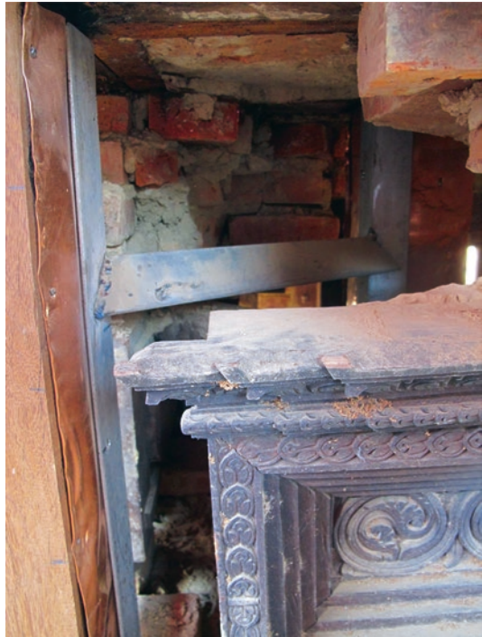
Fig. 10.4 Use of cement and steel frames visible within reconstruction of the Lakshmi Narayan Temple by KVPT in Hanuman Dhoka's Durbar Square (Photographed in December 2016)
