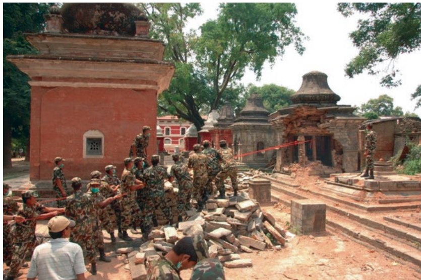
Fig. 10.2 Military personnel deliberately collapsing a damaged shrine at Pashupati (Source: Image Courtesy of Pashupati Area Development Trust)
