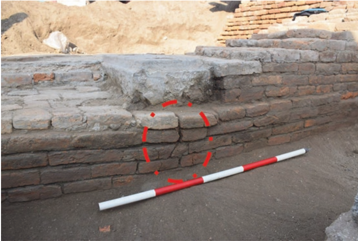
Fig. 10.13 Vertical cracks below a double saddlestone in the east facing elevation of the western north–south foundation alignment of the Kasthamandap
