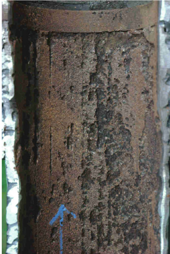
Fig. 4 CO 2 internal corrosion on carbon steel pipe
