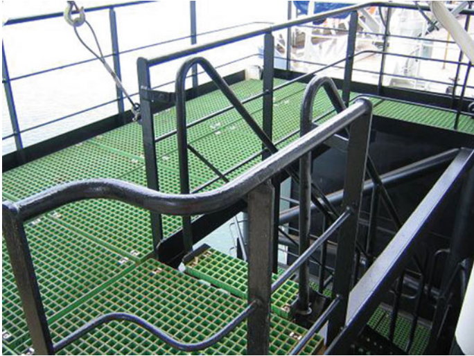
Fig. 14 Molded grating on offshore structure
