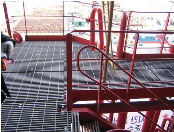
Fig. 13 Pultruded phenolic grating on offshore structure
