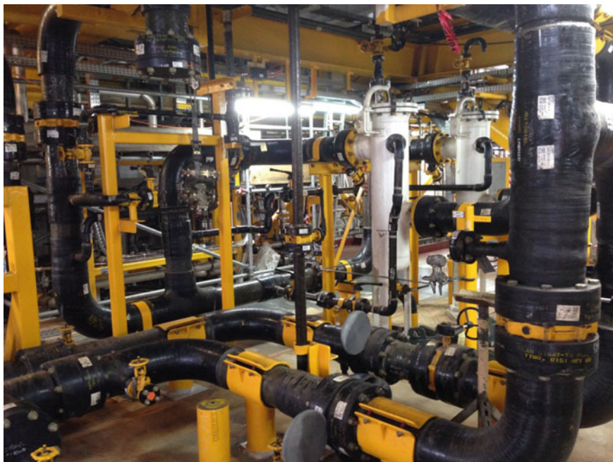
Fig. 7 Fire fighting system network on an offshore facility (Courtesy of SBPI)
