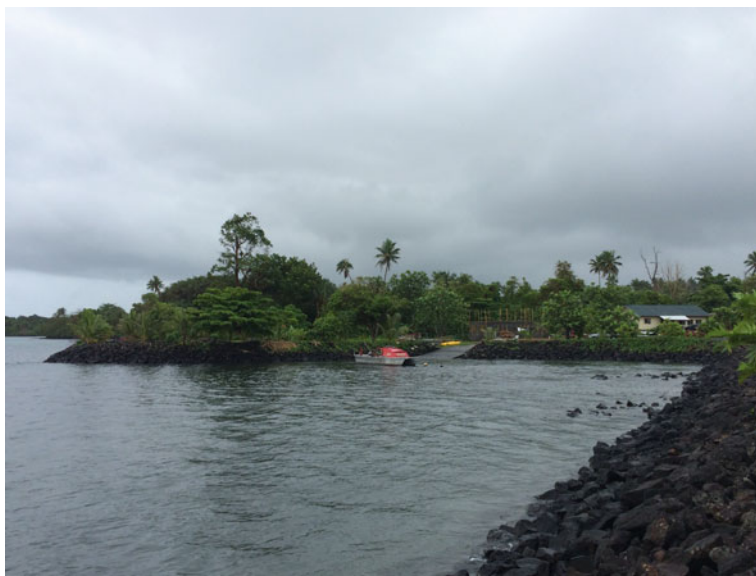
Fig. 16.4 Coastal seawall of Poutasi village on south coast of Upolu island. Photo credit Miguel Extetban, 2015
