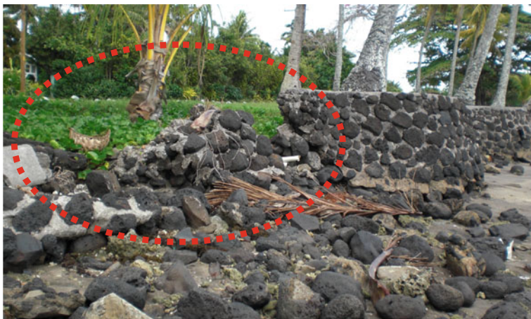
Fig. 16.5 Damaged coastal seawall in Vaiala. Photo credit Tomoya Shibayama
