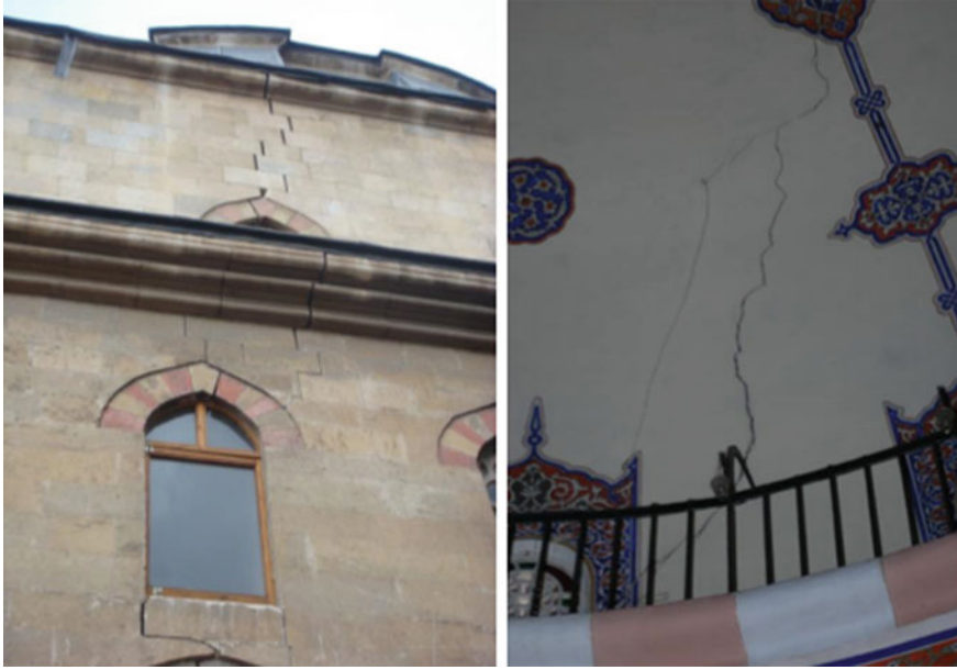
Fig. 11. Wall and dom cracks observed in the Cenab-ı Ahmet Pasha Mosque due to settling/sinking at different times [13]
