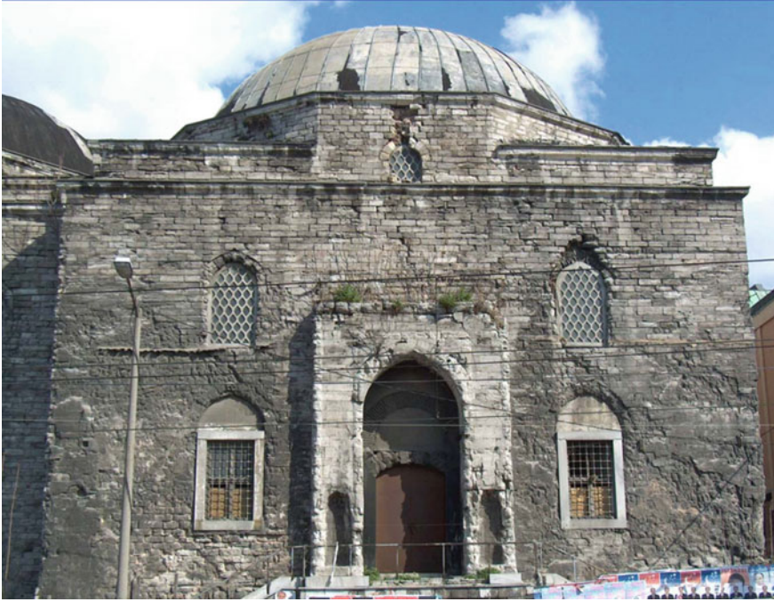
Fig. 1. Cracks visible on the main outer wall of a historic mosque [4]
