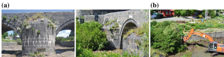
Fig. 8. a Plants seen from the bridge before restoration, b Cleaning of plants during restoration
