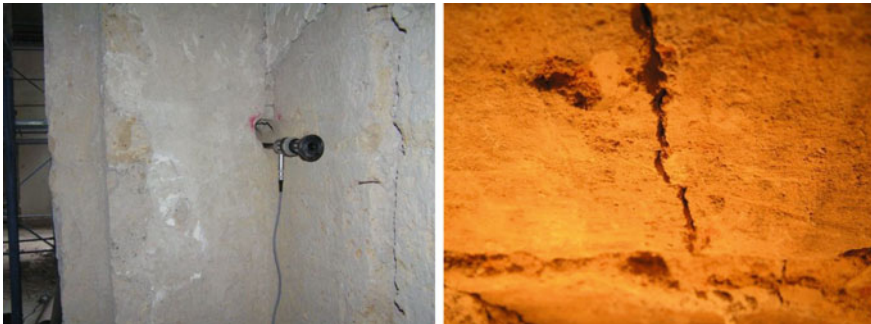
Fig. 4. Damage assessment using the endoscopy method
