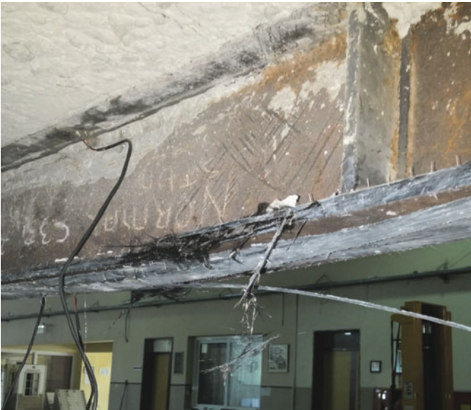
Fig. 12. Rupture of CFRP in strengthened sample
