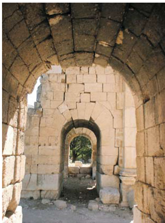
Fig. 3. Joint dislocations in a vault [3]
