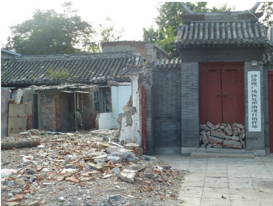
Fig. 15.3 Demolition of the Bell and Drum towers square, September 2014. © F. Graezer Bideau
