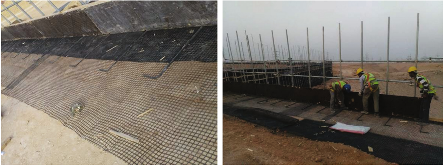
Fig. 10. Installation of anchor dowels/bars on top of wrapped back portion prior to installing subsequent reinforcement layer
