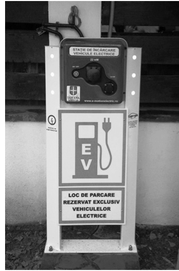
Fig. 6. Exterior semi-public fast charging station [7].
