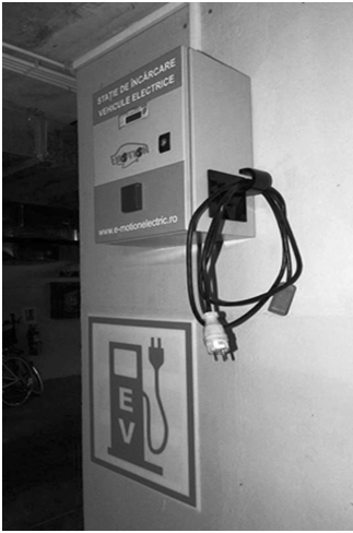
Fig. 5. Interior public charging station [7].
