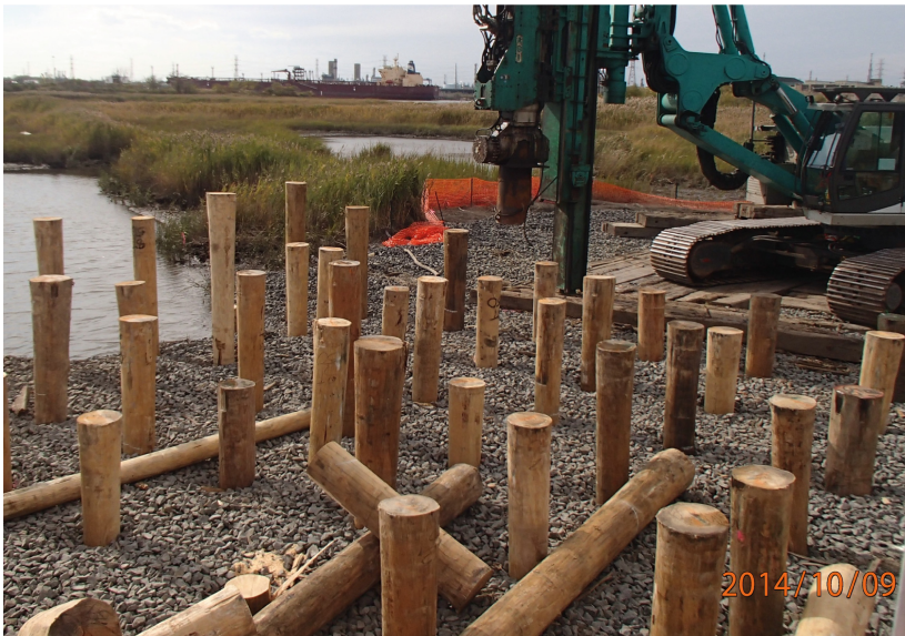
Fig. 8. Installation of timber piles during the construction of the geogrid-reinforced pile-supported embankment
