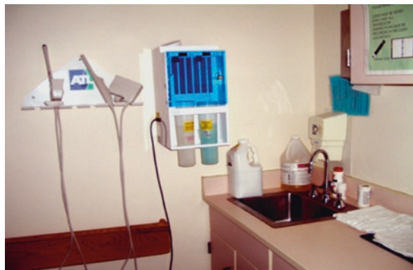
Fig. 15.17 Mounted portable HLD soak station
