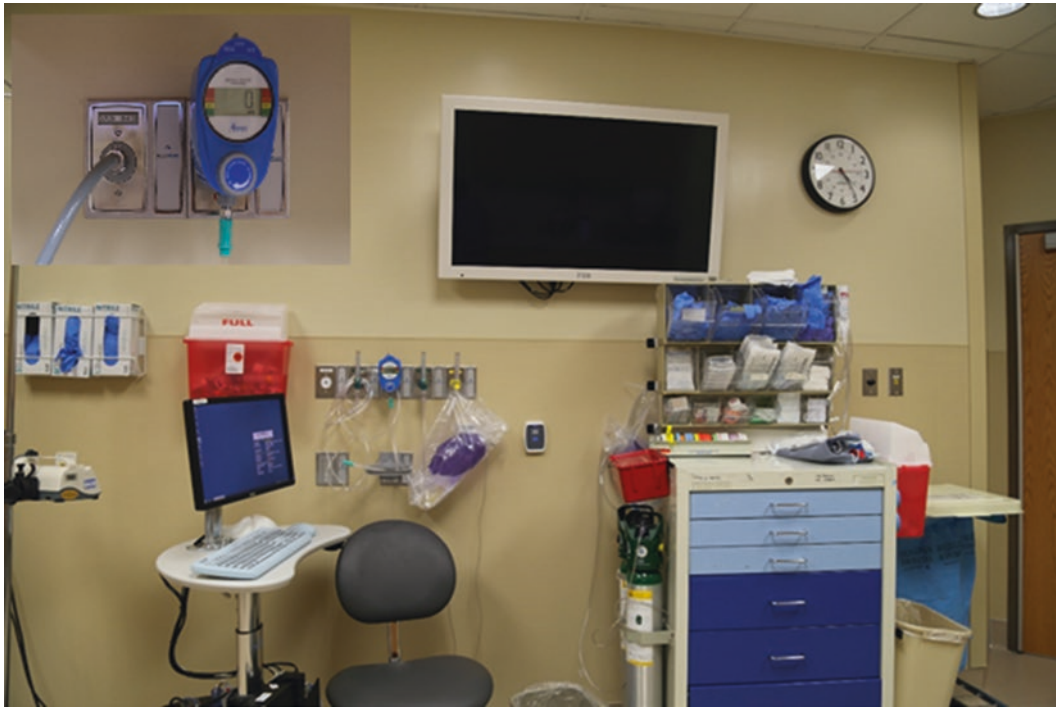
Fig. 44.3 Endoscopy suite with large adjustable wall monitor, wall-mounted air, vacuum, oxygen, and pipe CO 2 (insert)
