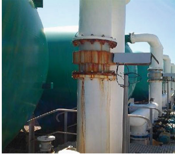
Fig. 3 Corrosion in sand filters
