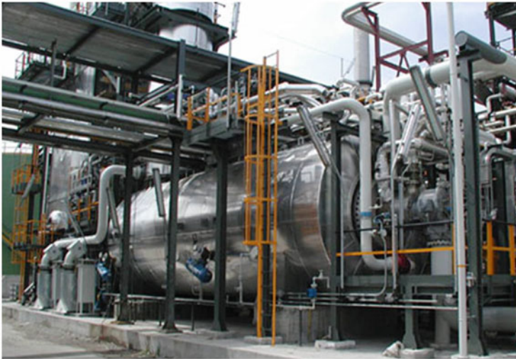
Fig. 3 System under study (Hydrogen sulfide tank)
