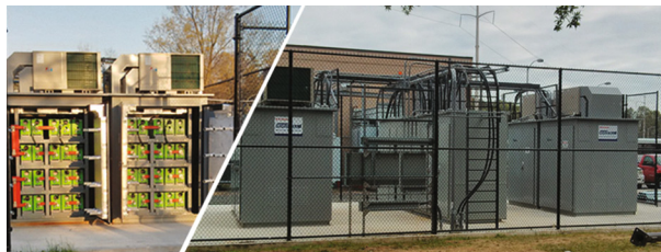
Fig. 1. GIGACELL batteries system. (Source: Kawasaki Rail Car [15])
