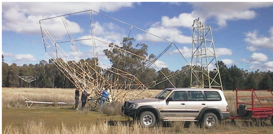
Fig. 19.99 The dismantling of one of the Radioheliograph antennas prior to its removal from the site. In the background on the left is one of the corner reflectors (Orchiston collection)
