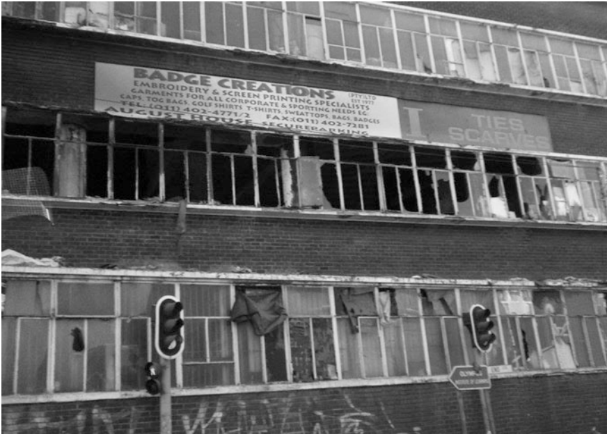
Fig. 4 Shot of one of the many “bad buildings” in Johannesburg’s inner city (Photograph by L. Burocco)
