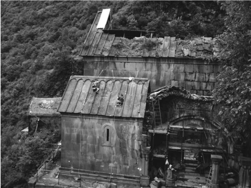
Fig. 2 The course for Ancient Masonry Restoration organized during the Preservation Training Project in Armenia was the occasion to preserve the roof of the gitz madur of Kobayr monastic complex (Lori region, Armenia), 2014
