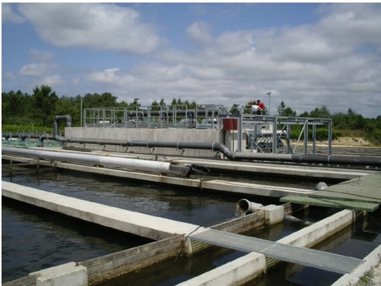
Fig. 38.6 Example of a large RAS (Recirculated Aquaculture System). The structure in the center of the photo is settled in between two series of raceways. It is mainly composed of biological filters and a depuration system to take out the nitrogen (fluidized beds). L' Esturgeonnière sturgeon farm, South West of France (credit P. Williot)
