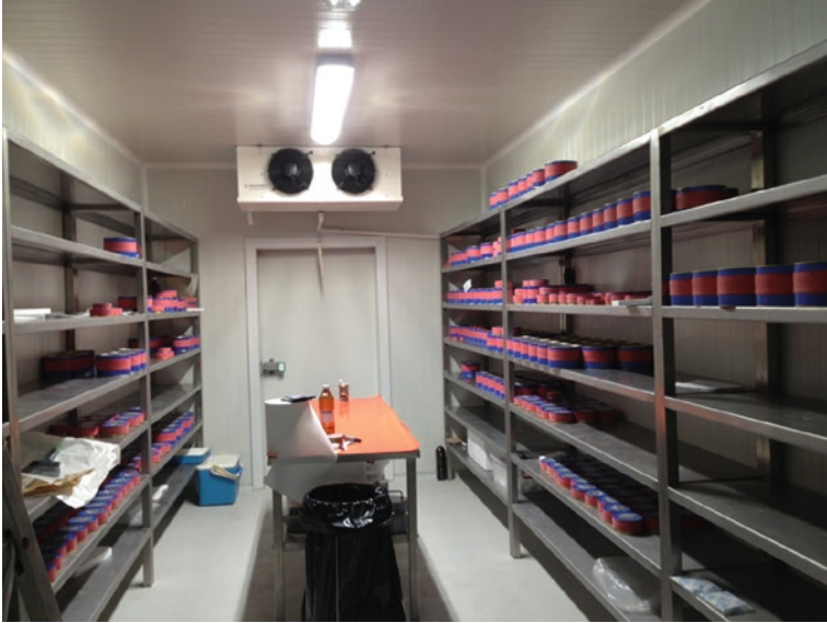
Fig. 38.22 Thermoregulated room for holding malossol-type caviar in Bulgaria. The two air conditioners in the top middle of the picture control the temperature (credit E. Galich)
