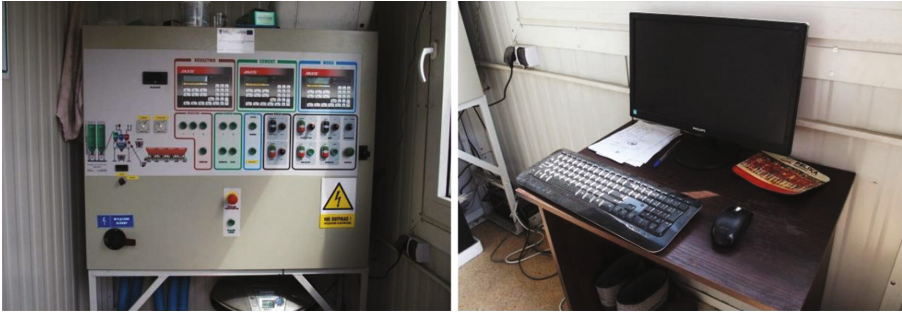
Fig. 5. Batching plant control panel [2]
