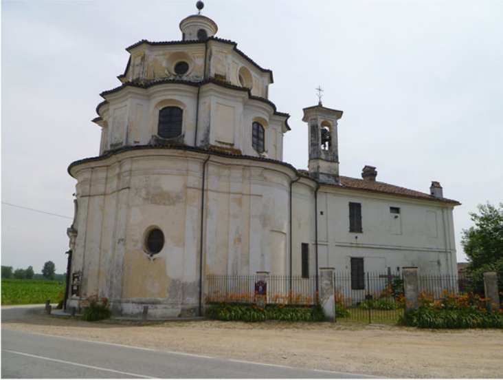
Fig. 10.1 The Santuario della Visitazione al Valinotto complex, north side. The main entrance is on the other side. Note, on the right, the sacristy (picture of the authors)
