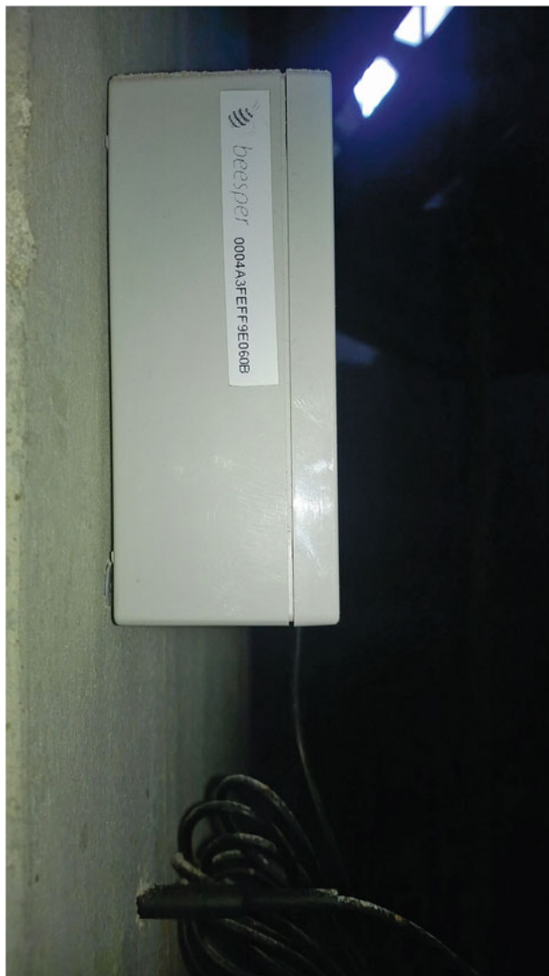
Fig. 10.6 Profile picture of a node with the sensor and, in the lower part, the contact sensor inserted in the wall
