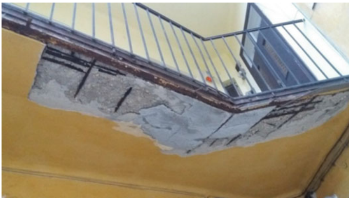
Fig. 13 Corrosion of the reinforcement rod
