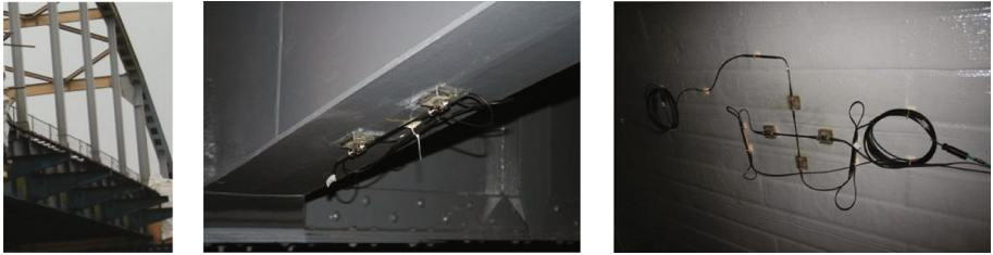
Fig. 6. Sideview cyclist path with sensor locations on the steel consoles and FRP composite bridgedeck
