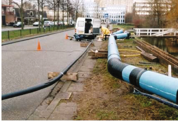
Fig. 1. Instrumented water transport pipeline
