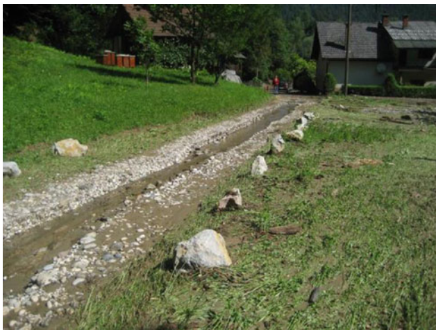
Fig. 7 The consequences of flooding it’s clearly visible; the torrent diverted from original channel and took the forest road as its riverbed (Kambič 2009)
