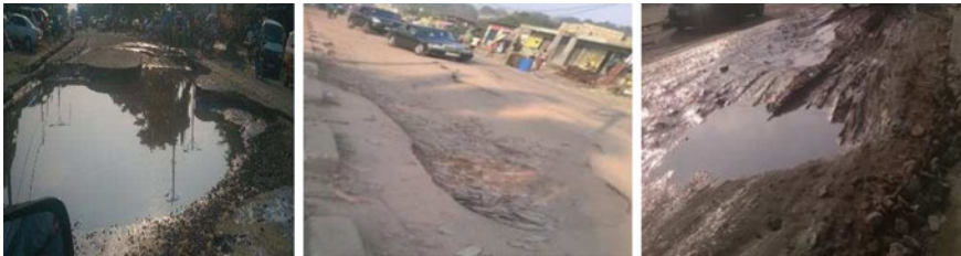
Fig. 6 Road potholes in Kinshasa (Photograph taken by A.K. Kayisu on 13 December 2015)
