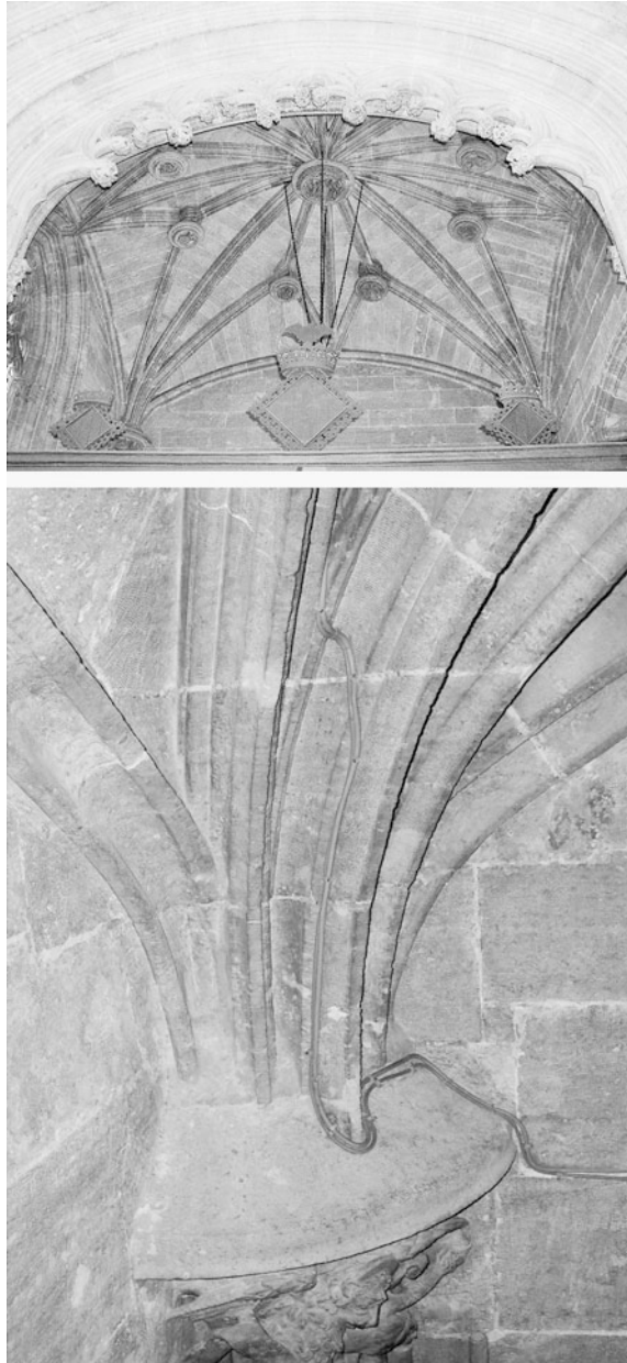
Fig. 5 Above, image of the Lonja chapel vault. Below, one of the spring, observe the profile of the wall-archs with diagonals and tiercerons. (Photo: E. Capilla. 31-10-2004)
