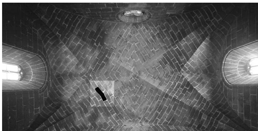
Fig. 10 View of a section of the dome of the Royal Chapel with an outstanding ashlar similar to that which has been analyzed in this article
