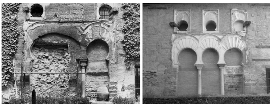
Fig. 8 Intervention on the tripartite gate of the north façade of the Plaster Courtyard
