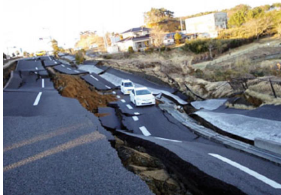
Fig. 2 Collapse of road surface due to ground motion (Route 6). http://www.thr.mlit.go.jp/road/jisinkannrenjouhou_110311/dourohisaijoukyou.pdf
