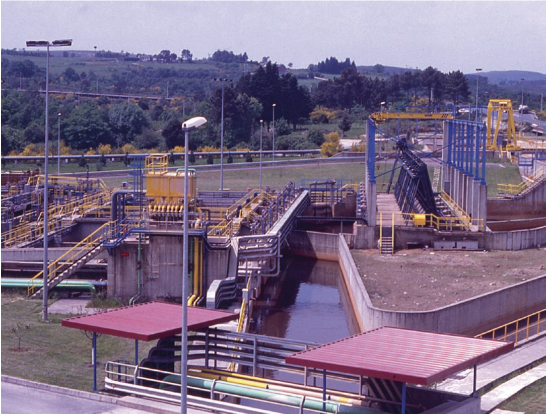
■ Fig. 7.17 Active water treatment plant near a coal mine
