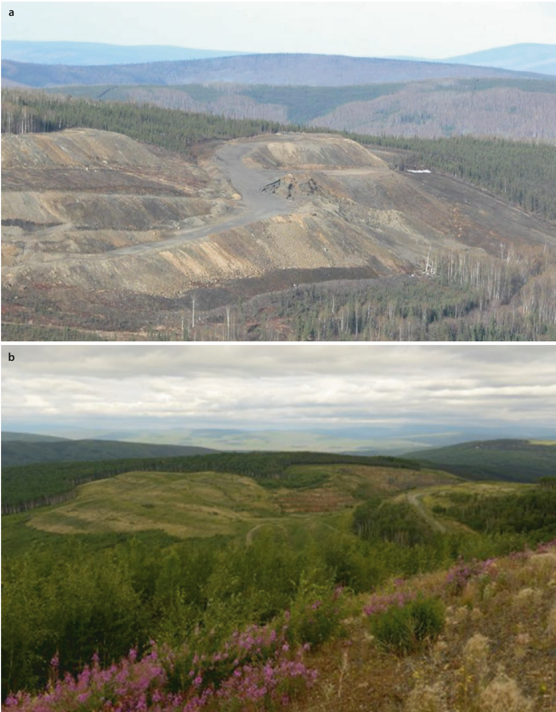
Fig. 7.44 a North Shepard Waste Rock Dump in 2005 prior reclamation (Image courtesy of Kinross Gold Corporation); b North Shepard Waste Rock Dump after reclamation in 2013 (Image courtesy of Kinross Gold Corporation)
