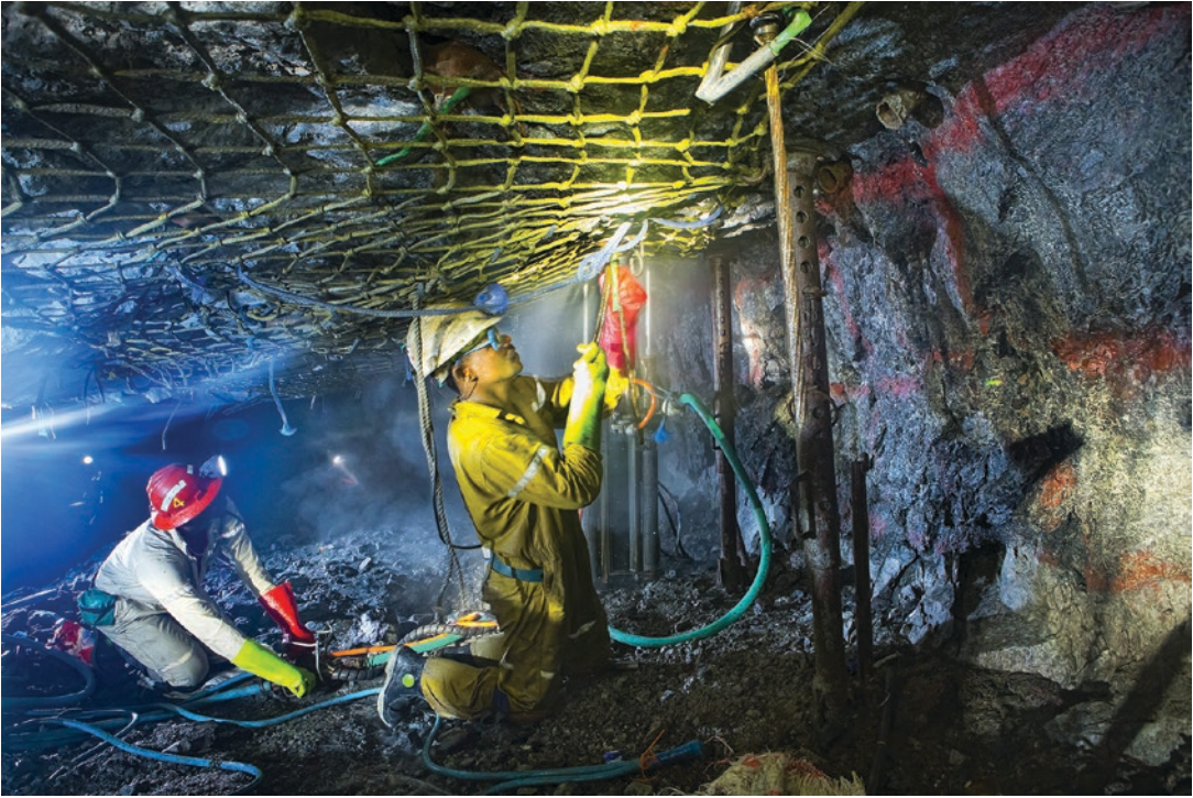
■ Fig. 5.55 Installing cable bolts at Dishaba Mine (South Africa) (Image courtesy of Anglo American plc)
