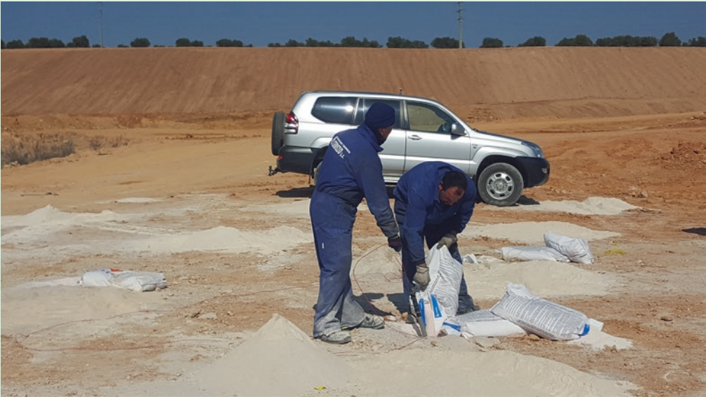
Fig. 5.80 Loading operation of ANFO nylon bags (Image courtesy of Octavio de Lera)
