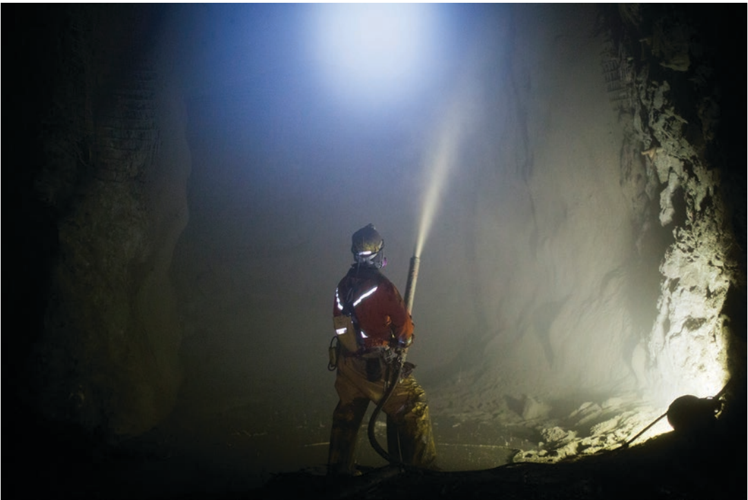
■ Fig. 5.56 Spraying shotcrete onto the walls of a drift underground at Snap Lake Mine (Canada) (Image courtesy of De Beers)
