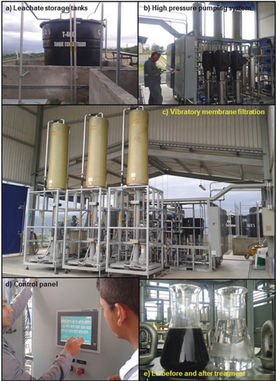
Fig. 5.8 Photographs of the Presidente landfill leachate treatment plant (Source: Photographs by the authors 2014)
