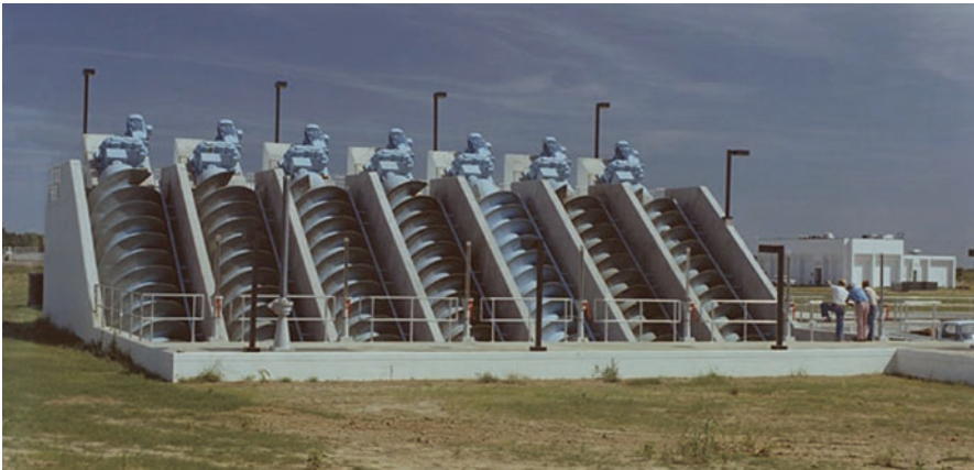
Figure 7 Wastewater treatment plant in Memphis, Tennessee, USA
