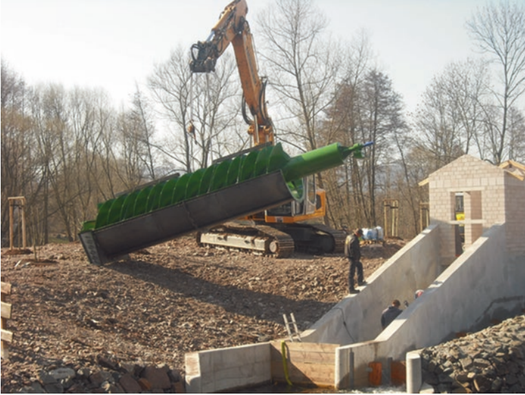
Figure 6 Installation of a hydropower screw on the River Apfelstädt in Herrenhof, Germany. The installation of a screw with an integrated steel trough takes only a few days and is very cost effective
