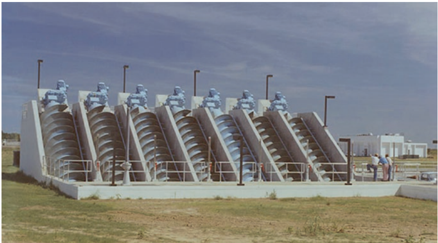
Figure 10 Memphis TN Wastewater Treatment Plant [Manufactured by Lakeside Equipment Company of Bartlett, Illinois, USA]
