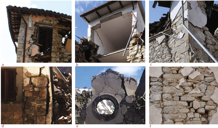
Fig. 6. The building before and after the earthquake October 30th, 2016.
