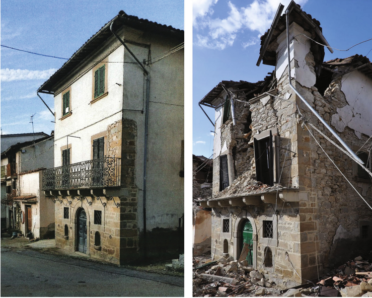
Fig. 5. a. Collapse of the central part of the façade with an example of well clamped angular masonry; b. Partial collapse of the structure in concrete blocks; c. Collapse of the angular masonry; d. Bulging angular masonry; e. The Church after the collapse of the roof; f. Masonry connected without the necessary clamping (evidenced by the lesion at the vertical plane of contact).
