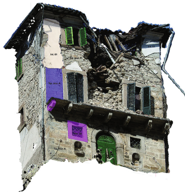
Fig. 1. Structure of the database with fields defining building type, coating, architectural details and damage and a semantic model, linked to database.
